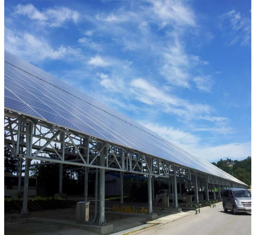
Young Dong Power Plant (1 MW)
